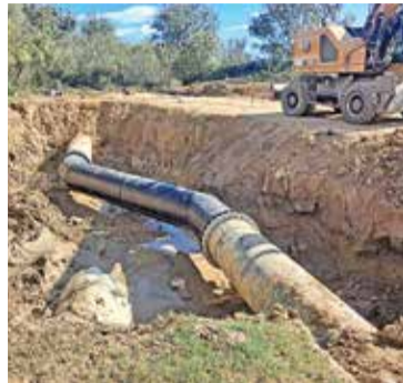
TRAM DE CANONADA A VILANOVA CACBG
